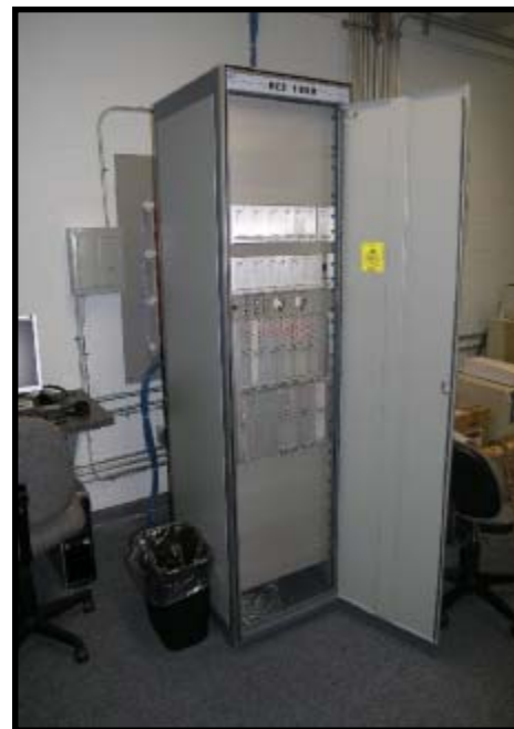
Refurbishing the PSO router saved more than $750,000. The router is the main computer system for directing incoming emergency calls for service.
