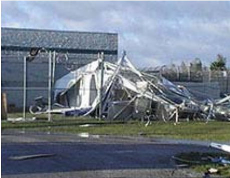
Fences needed to be replaced
